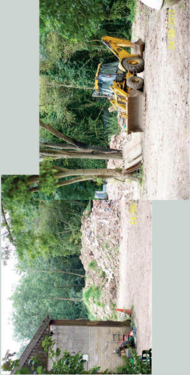
Fig 9 : Unauthorised waste deposit, transfer & disposal – 2012. Skips & waste cleared, just the hardcore remaining.
